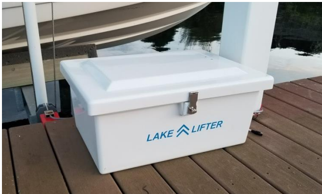
Install both batteries, control box, battery connectors, and excess wiring in the fiberglass battery box
